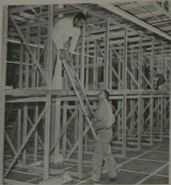
SIX DAYS and over 8 1/2 miles of AIM framing triples skid storage in an AIRsearch Manufacturing Company warehouse.
